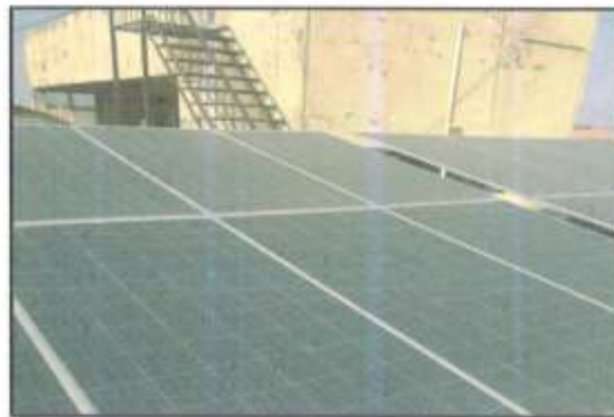
Photograph of Roof Top Solar PV Plant:
