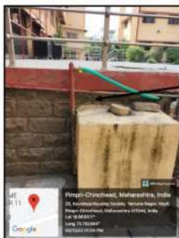
Photograph of Rain Water Management Recharging Well Section:
