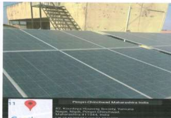
Photograph of Roof Top Solar PV Plant:
