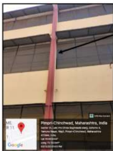
Photograph of Rain Water Management Pipe:
