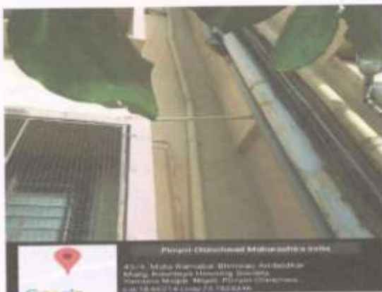
Photograph of Rain water Harvesting Pipe:
