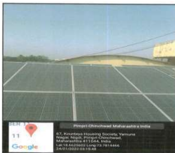
Photograph of Roof Top Solar PV Plant:
